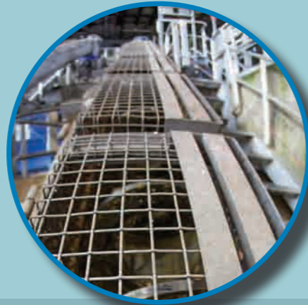
Screening is the first line of wastewater treatment. Here, screens at the Mangere plant intercept solid debris from raw wastewater. We use treated wastewater to clean these screens.
